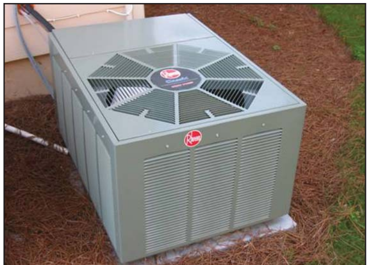
Figure 12.21. External Air-conditioning Condenser Unit
