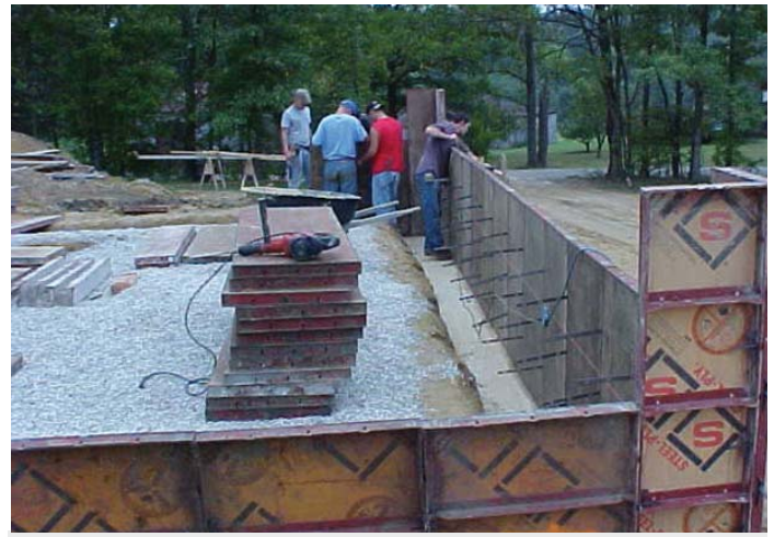
C. Concrete will be poured into this form on top of the footer to create the foundation of the home. Again, reinforcing rods are added to ensure that the concrete has both lateral strength, as well as the strength to support the home. Once the concrete has hardened and becomes seasoned, the forms will be removed to reveal the finished poured concrete foundation over the perforated drainage pipe. Not shown is a newer technique of using insulating polystyrene forms and ties in a building foundation.
