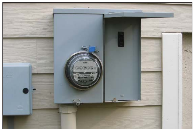
Figure 11.15. External Power Shutoff and Meter
