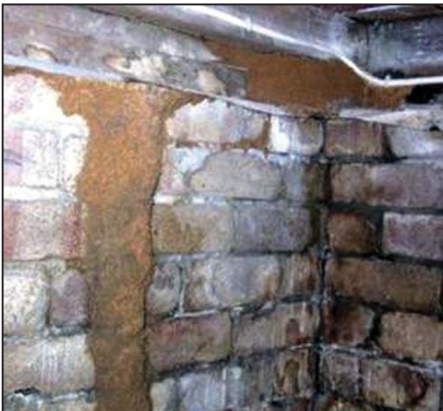
Figure 4.19. Termite Mud Shelter Tube Constructed Over a Brick Foundation [14]
