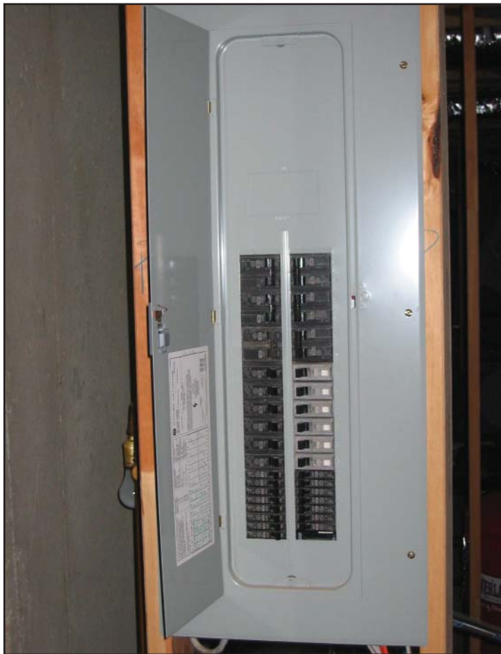
Figure 11.14. 200-Amp Service Box
