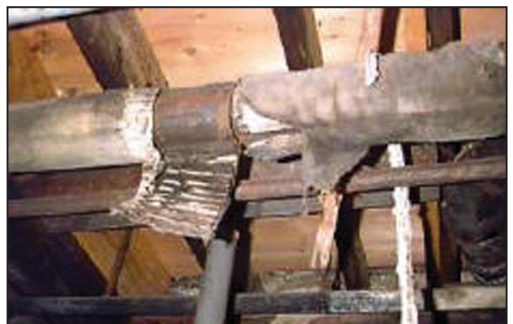
Figure 12.6. Heating Ducts Covered With Asbestos Insulation
