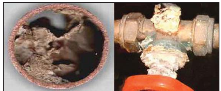
Figure 7.6. Corrosion in Piping Resulting From Galvanic Response
