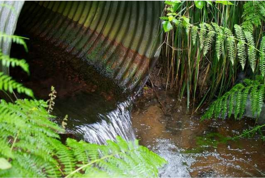
Perched culvert, impassable to small aquatic organisms. - Sam Beebe
