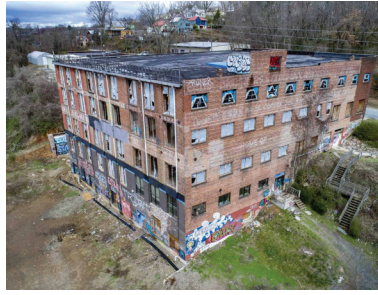
Run-down, poorly maintained
