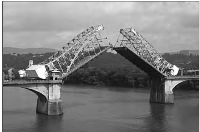
Figure VII-03: Photograph of the Market Street Bridge (#85, 33-SR008-09.53) in Chattanooga during a routine inspection during which the bascule lift is activated and the leaves opened.
