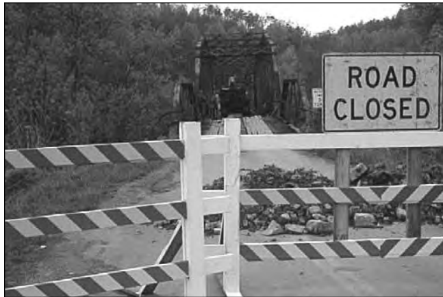
Figure VII-01: Photograph of the Massengill Bridge in Anderson County as demolition begins (#87, 01-A0088-03.53).
