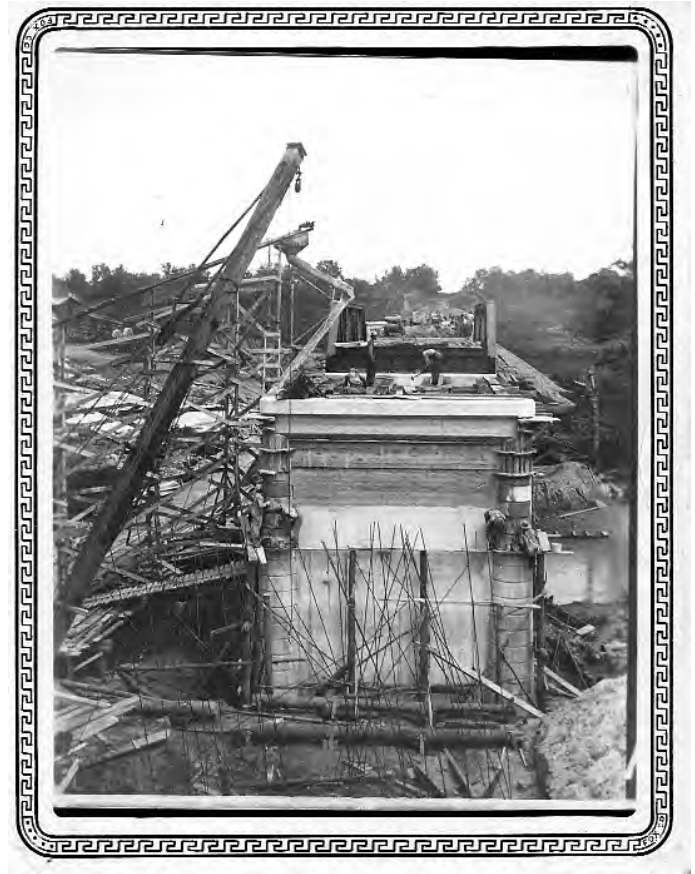
Figure II-47: Road and Bridge Construction Scenes in Tennessee. Construction crews working on a bridge spanning Beech River, State Route 69 between Decaturville and Parsons, Decatur County, 1929 (top right); Near Nobusiness, Campbell County, 1927 (bottom); a wheel scraper crew working in Haywood County in 1922 (top, next page); and road construction near Peabody, 1927 (bottom, next page) (TDOT Photo Collection).
