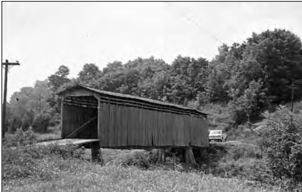
Figure II-18: Historic Postcard view of the Bible Bridge in Greene County, now the focal point of a small county park, (#109, 30-A0906-00.01) (Author's Collection).
