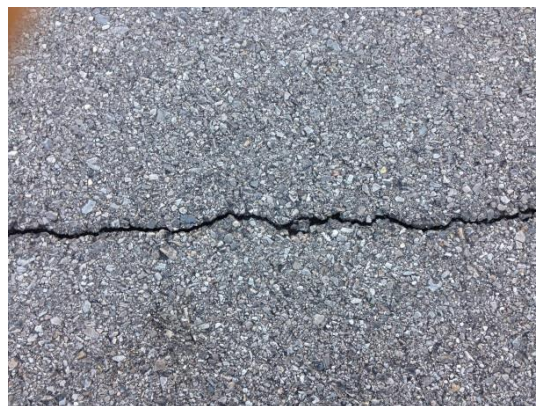
Figure 7- 1 Original image of a crack
