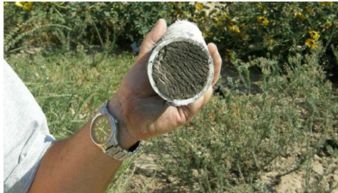
Figure 2-2. Example of a drain clogged with fine sediments from the drainage layer. From Bhattacharya et al., (2009).
