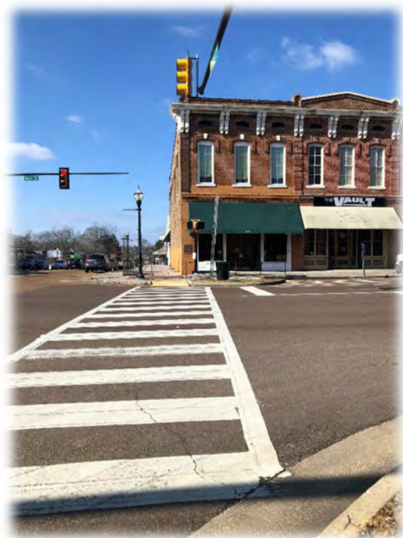
Crosswalk at Main Street Pedestrian Signal Aligned Improperly
