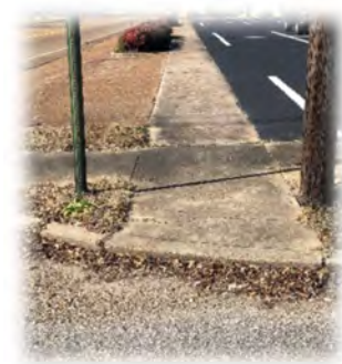
Missing Ramp on Side Road
