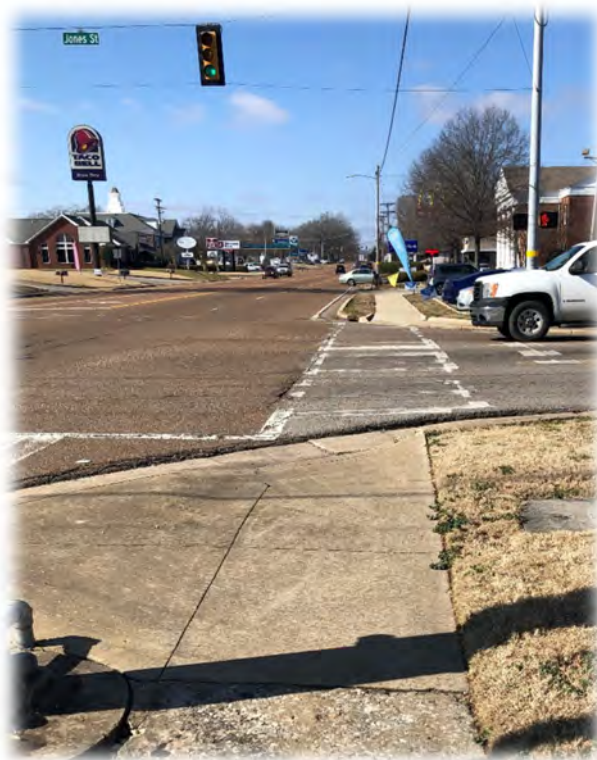
Crosswalk at Jones Street Faded Striping
