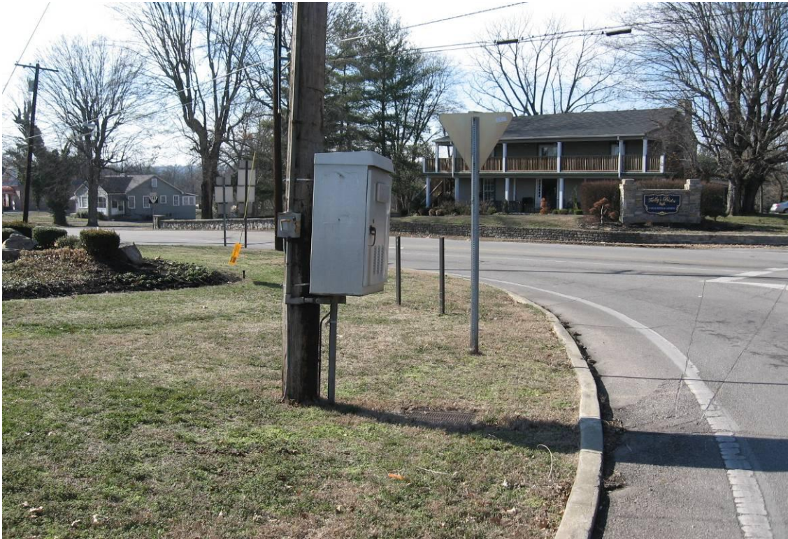
Signal Pole and controller box located in southeastern quadrant
