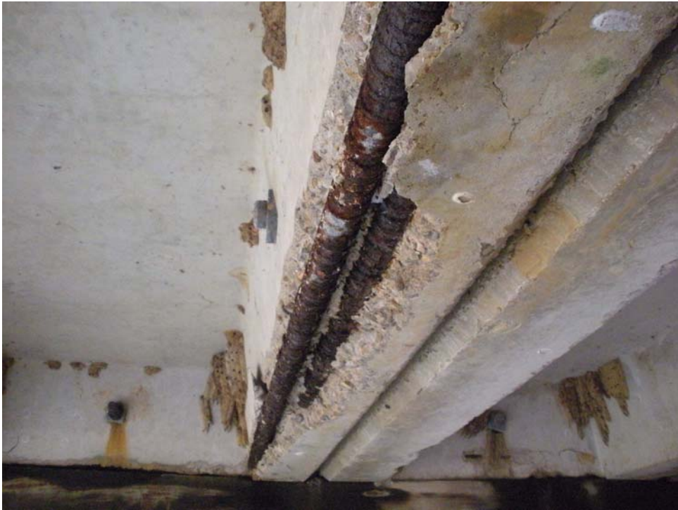
Concrete Channel Section (Exposed Rebar)
