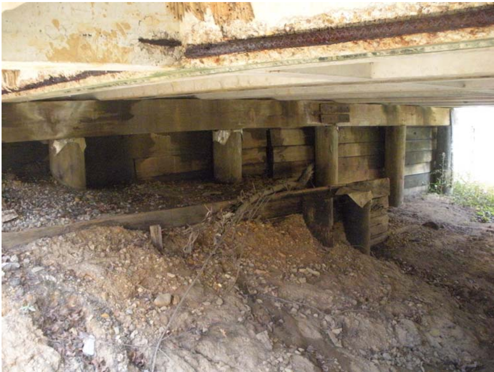
Bridge Abutment (More Exposed Rebar)
