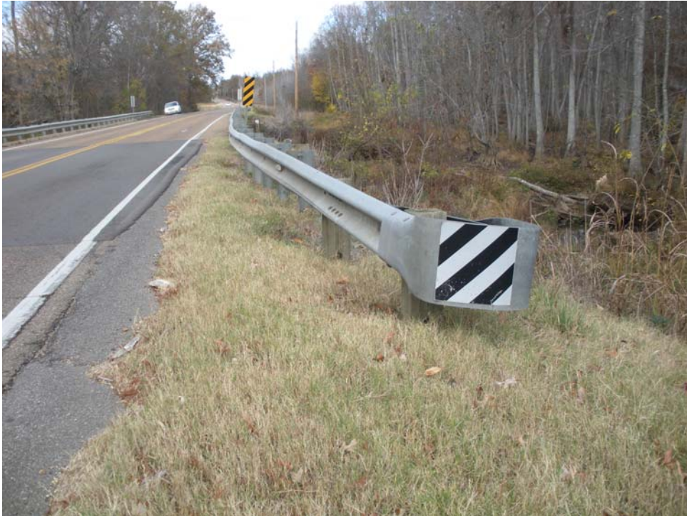
Guardrail End Treatment
