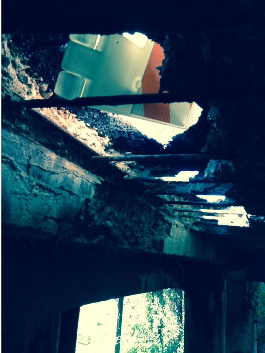
Hole on Bridge Deck with Exposed Rebar
