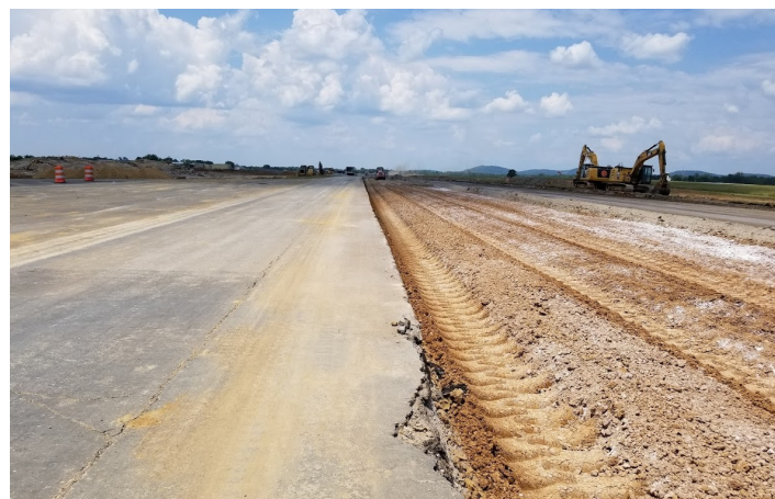
Shelbyville Municipal Airport, Bomar Field, in Shelbyville, TN during major runway reconstruction and RSA improvements.
