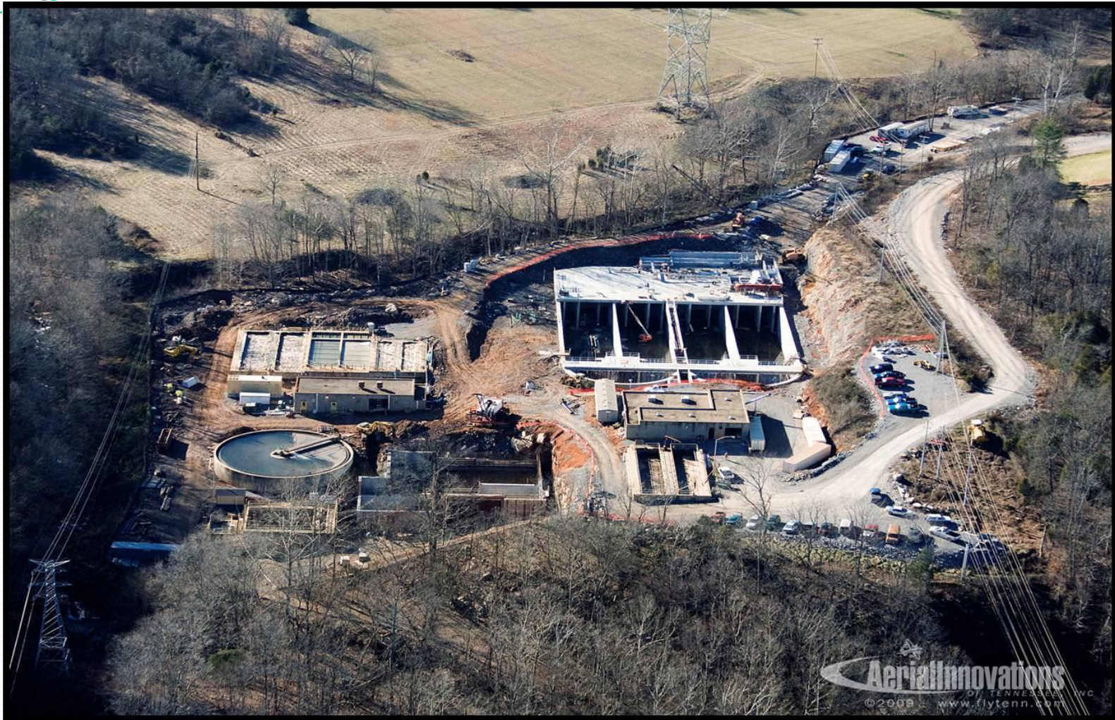
Regional Wastewater Treatment Plant Expansion $24M Expansion form 2.25 to 6.0 MGD
