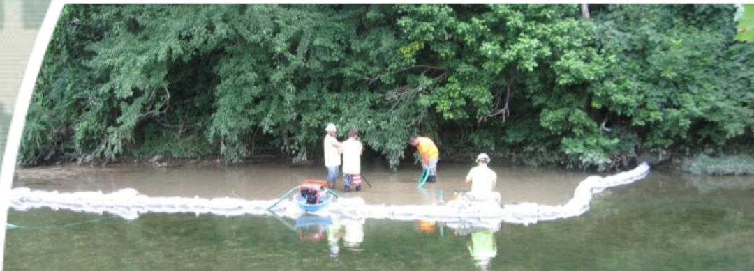
Mill Creek HDD Hydraulic Fracture Clean-up
