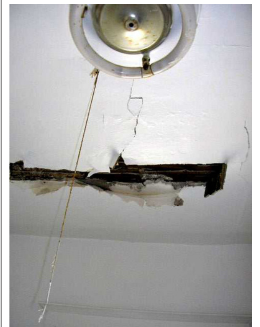
FIGURE 8.4 Example of structural deficiency needing repair prior to work.
