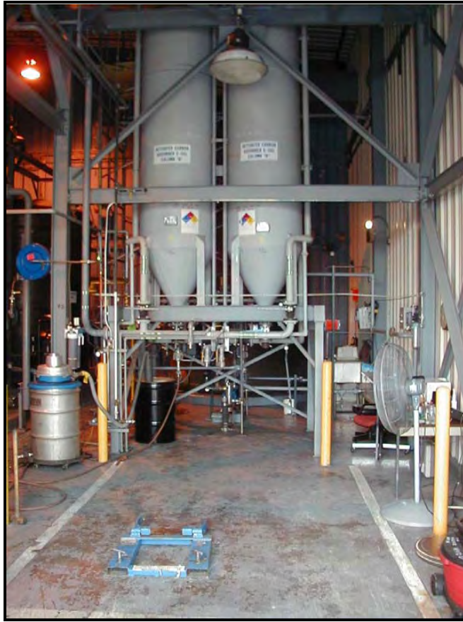
Fig. A.3. GWTF located in Bldg. 9616-7.
