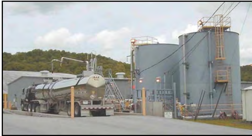
Fig. A.2. Leachate Storage Facility.
