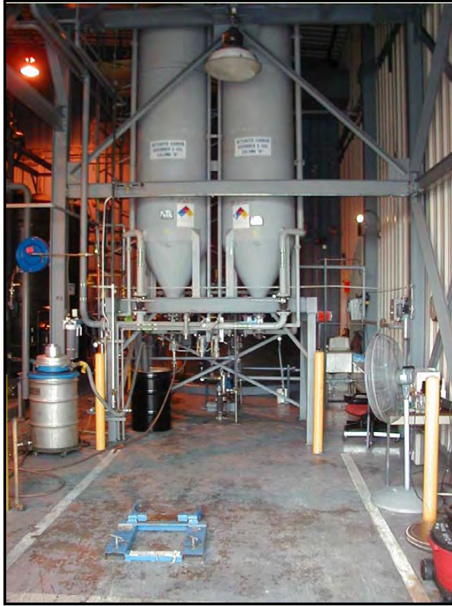
Fig. A.3. GWTF located in Bldg. 9616-7.
