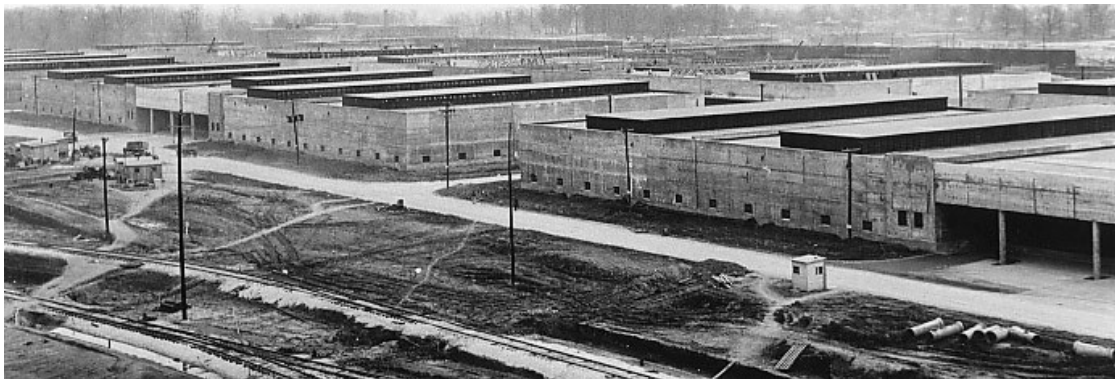
Figure 22. Memphis General Services Depot under construction (Memphis Depot Business Park website http://www.memphisdepot.net/history.htm ).
